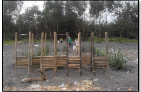
Figure 6. Apo-apo is installed in the frontage to decrease the coming wave power
